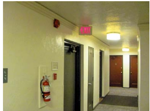
Typical corridor lighting and fire alarms
