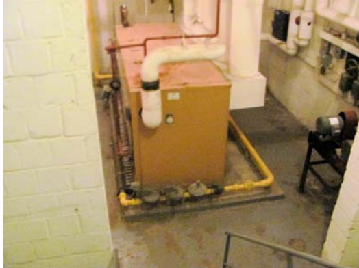
View of gas boiler
