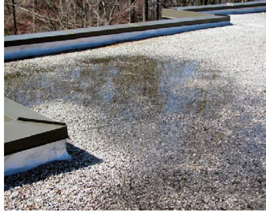
Water ponding on roof
