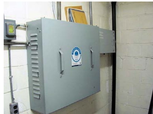
Elevator electrical controls
