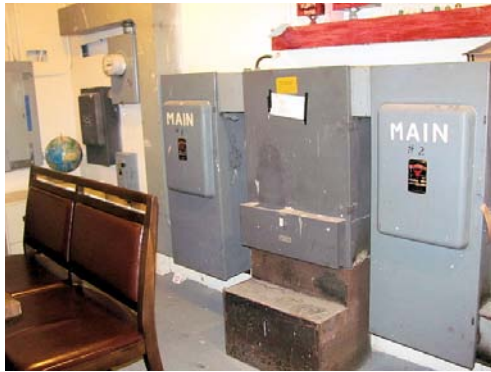
Main disconnect panels
