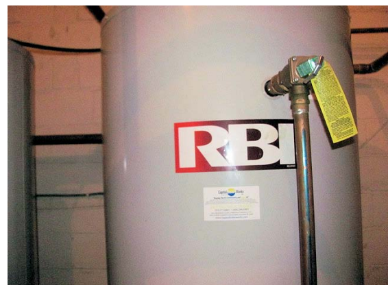
Pressure release valve on new 200 gallon hot water storage tank
