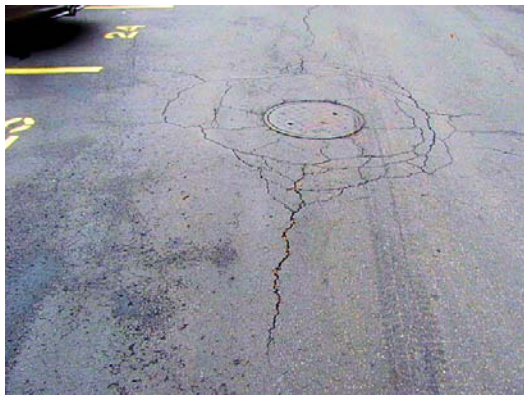
Open cracks and alligating surface
