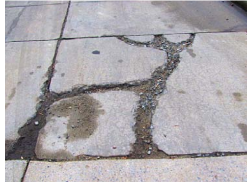
Damage concrete apron at parking lot entrance
