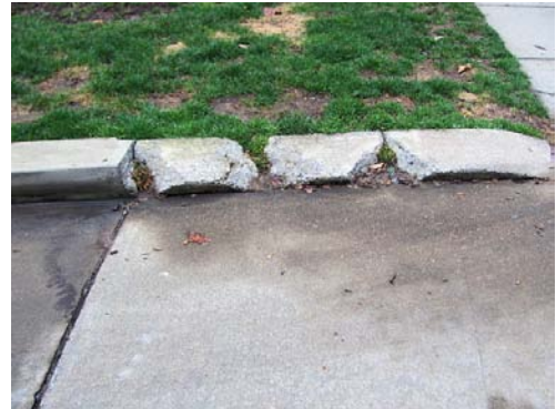
Broken curb at entrance apron
