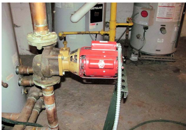
View of two gas water heaters and circulator pump at storage tank
