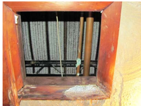
Pin hole leak in copper pipe
