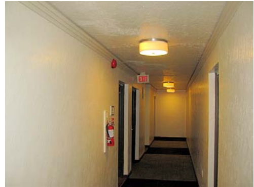
Typical corridor lighting, fire pulls, bell and exit light
