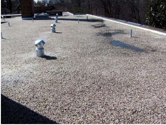
Water ponding on roof
