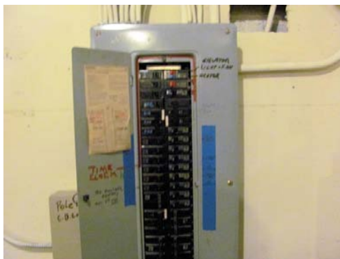
Common area distribution panel
