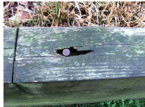
Deterioration in wood section
