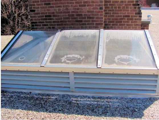
View of skylight with condensation between the plastic panels
