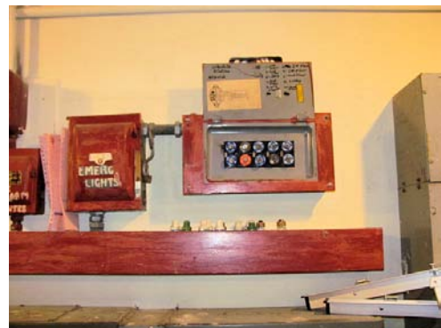
Fuse panels controlling the emergency lights and fire alarm system
