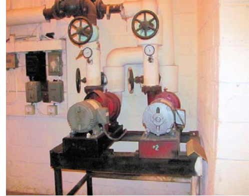
Hydronic circulator pumps
