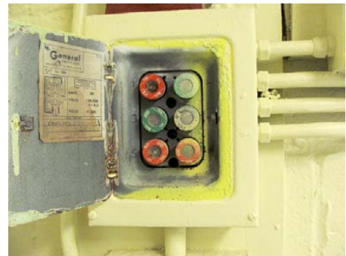
Fuse panel in laundry room
